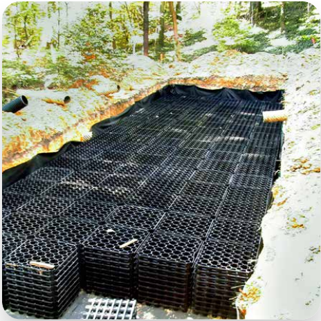
Underground Detention Basin
