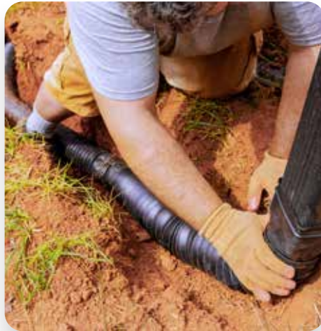
Downspout Catch Basins
