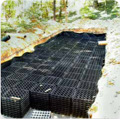
Underground Detention Basin
